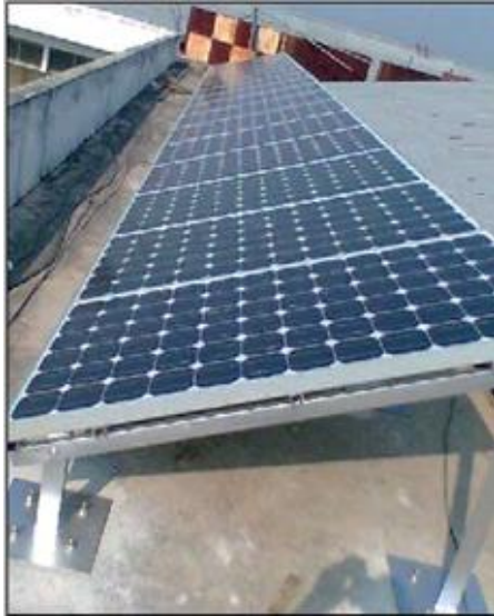
Figure 2. Conversion Efficiency 14%, 16 × 160 W Modules Mounted at the Roof-top of the Class Room
