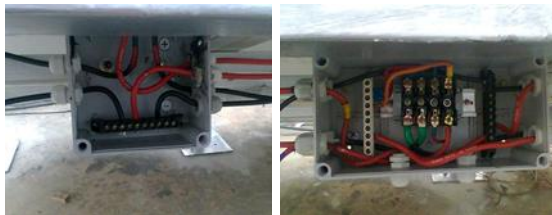
Fig.3 Wire Connection in Connection Box and Fuse Box
