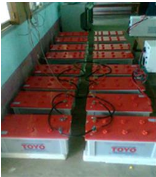
Fig.5. 200Ah batteries for storing the charges for later use
