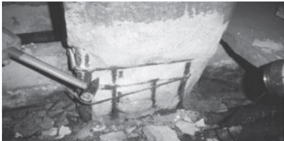
Figure 11 - Steel reinforcement after 10 years in closed area
