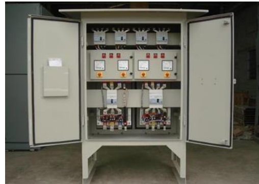
Plate 1: Electrical Feeder Pillar
