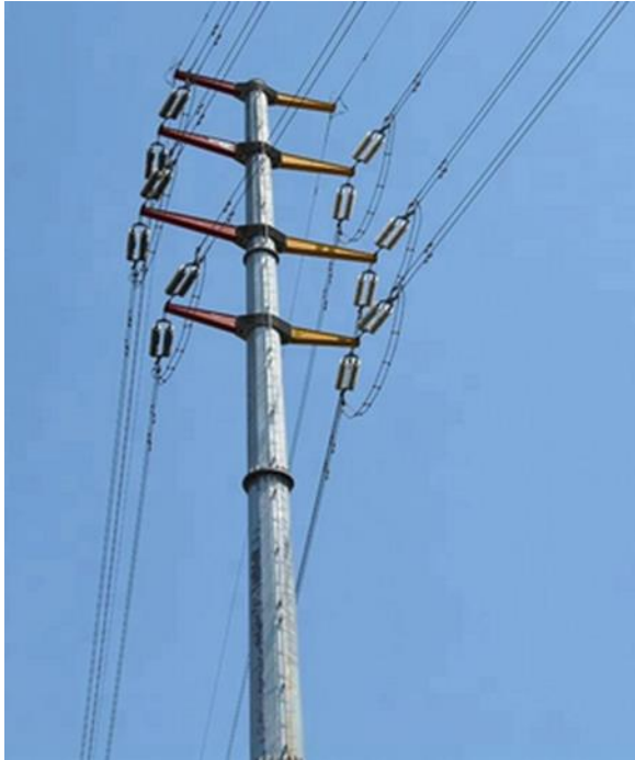
Figure 1.1: A typical 132kv Transmission line steel Tubular pole
