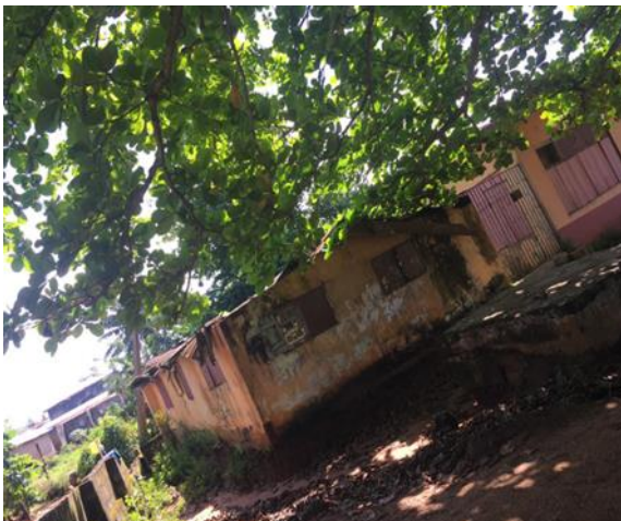
Picture 4: Showing Existing Condition of A Public Primary School in the remote Area of Yewa South, Ogun State.
